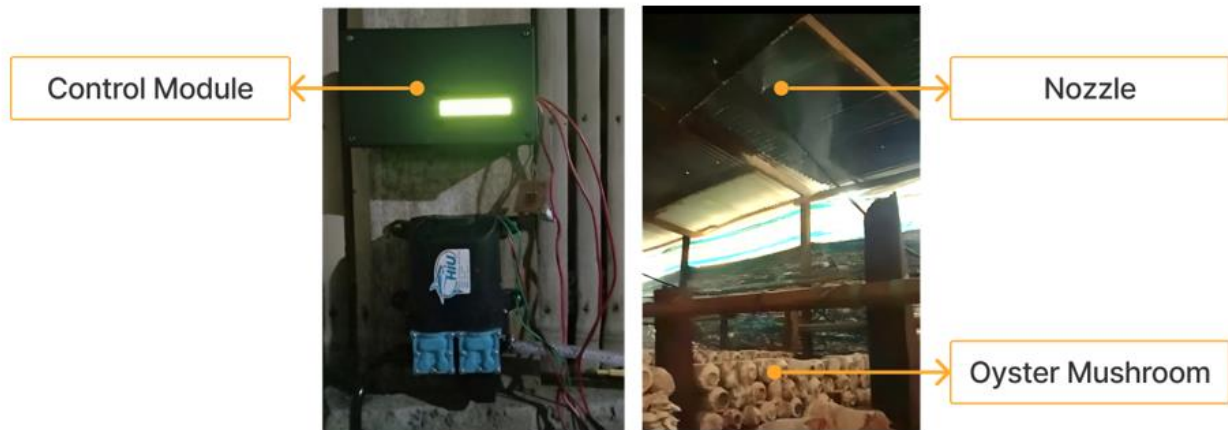
Figure 5. Installation of the device in mushroom cultivation
